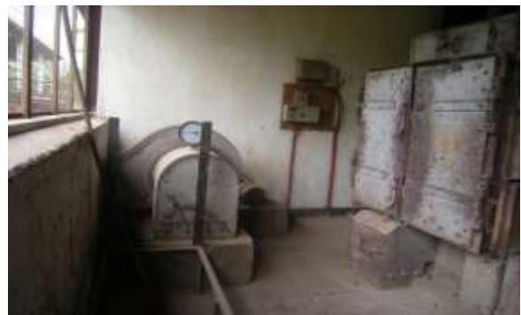
Plate 4 Faulty ID temperature and inadequate space for cleaning tubes
