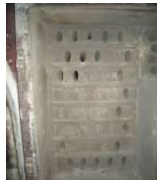
Plate 6 Blocked oval tubes
